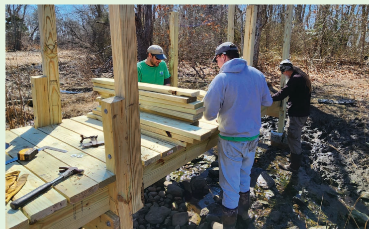
From left: Conservation staff Mike Cavaliere, Lincoln Dark, and Joe Metzen at work in March on the new foot bridge.
